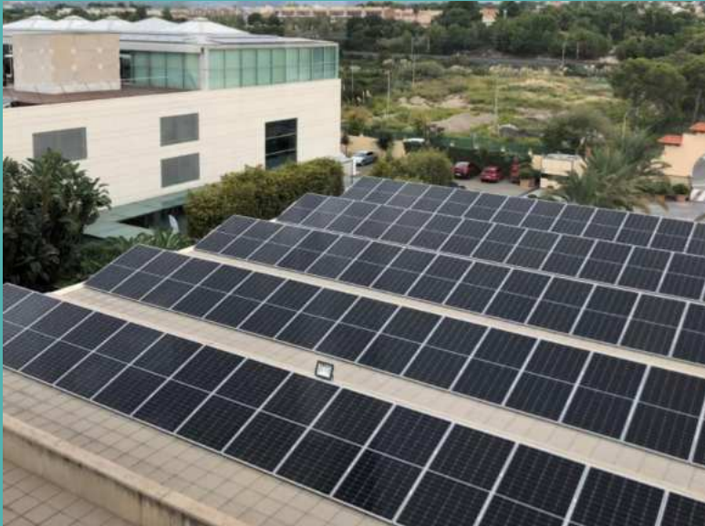
Photovoltaic panels that will generate 15% of the energy consumed by the hotel.
